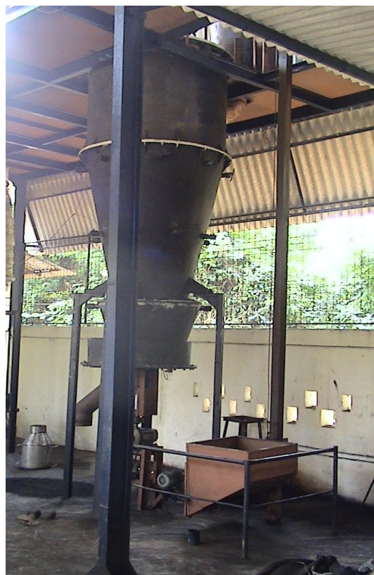
Fig. 1. Carbonizing pilot plant: An overall view
