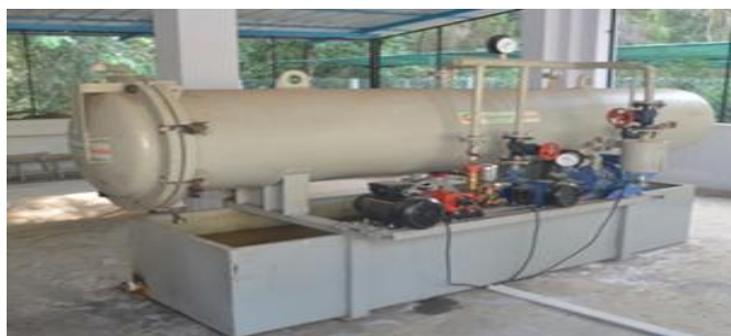
V P I Treatment Plant
