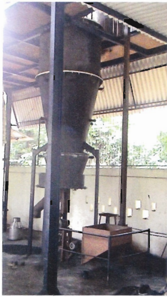
Fig. 8. Carbonizing pilot plant: An overall view
