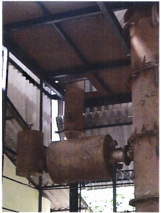
Fig. 37. Flue gas burning furnace attached to the FBR
