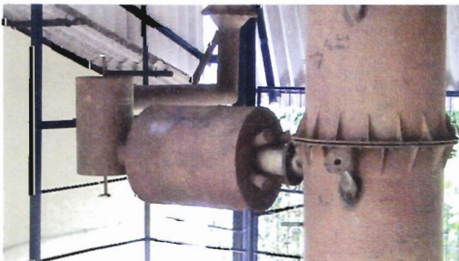
Fig. 39. Internal view of the super heater
