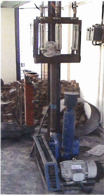
Fig. 36. Air compressor with pressure gauge
