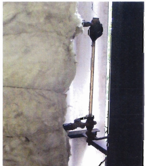
Fig. 45. Water level view glass in the boiler
