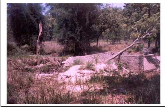
Broken check dam in Nellur thodu (Muthanga range- Wayanad WLS)
